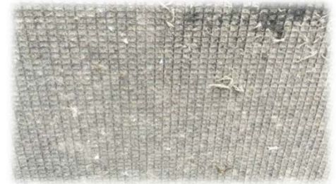
2 week installation trial on a MCC Chiller at Palm Paper shows the amount of paper fiber & debris PreVent® stopped from going into the coils.
