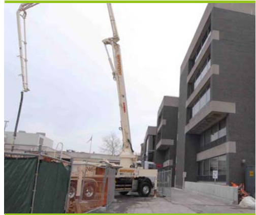
Construction begins just 30 feet away from the fan coil air intakes.
