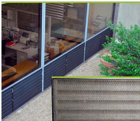
Air intakes and fan coil units are located below and just inside windows.
