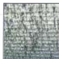
Flattened intake fins block optimal air flow.
