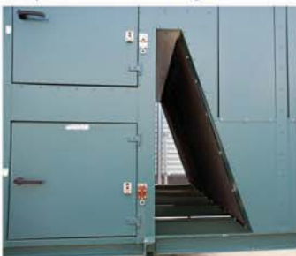
PreVent works well keeping hard to access air intakes clean. Debris is easily brushed off with a broom.
