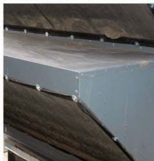
Debris like cottonwood can be captured before it enters the system or gets embedded in fins.
