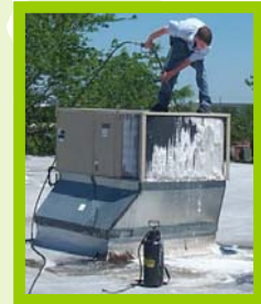
EXTENSIVE LABOR & CHEMICALLY CORROSIVE CLEANING
