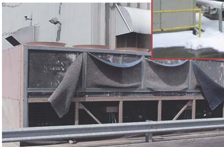
A 200 ton chiller before and after proper air intake filtration.
